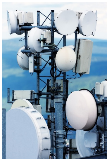
Telecom antenna tower
